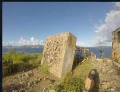
Buck Island Weather Station, St. Thomas, tower toppled but instrument not silent:
