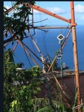
Crown Mountain Weather Station, St. Thomas, damaged and silent
